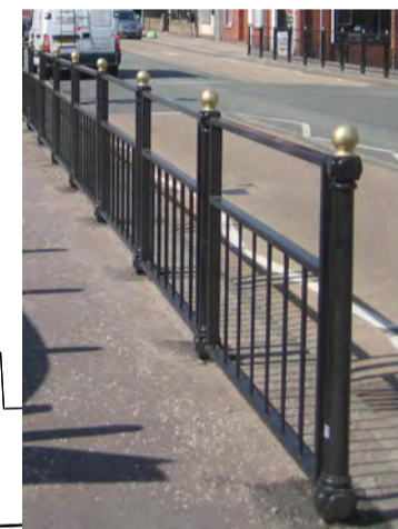
Replace old galvanised barriers with black and gold type and de-clutter signage. Repair broken knee rail.
