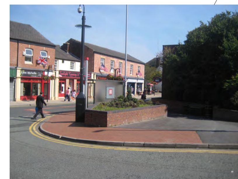
Site on corner of Hill St - Removal of raised planter, improvements to wall at rear, repaving of area with integral maze pattern
